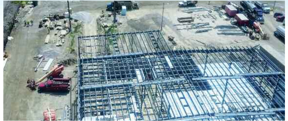
A view from the new tower at the Magnus International Group site shows the progress on the rest of the construction project, where IBEW Local 673 members and travelers are working.
