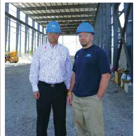
Owner John Darby (left) and Local 41 Steward Ron Bailey stand in front of Niagara Transformer's building expansion.
